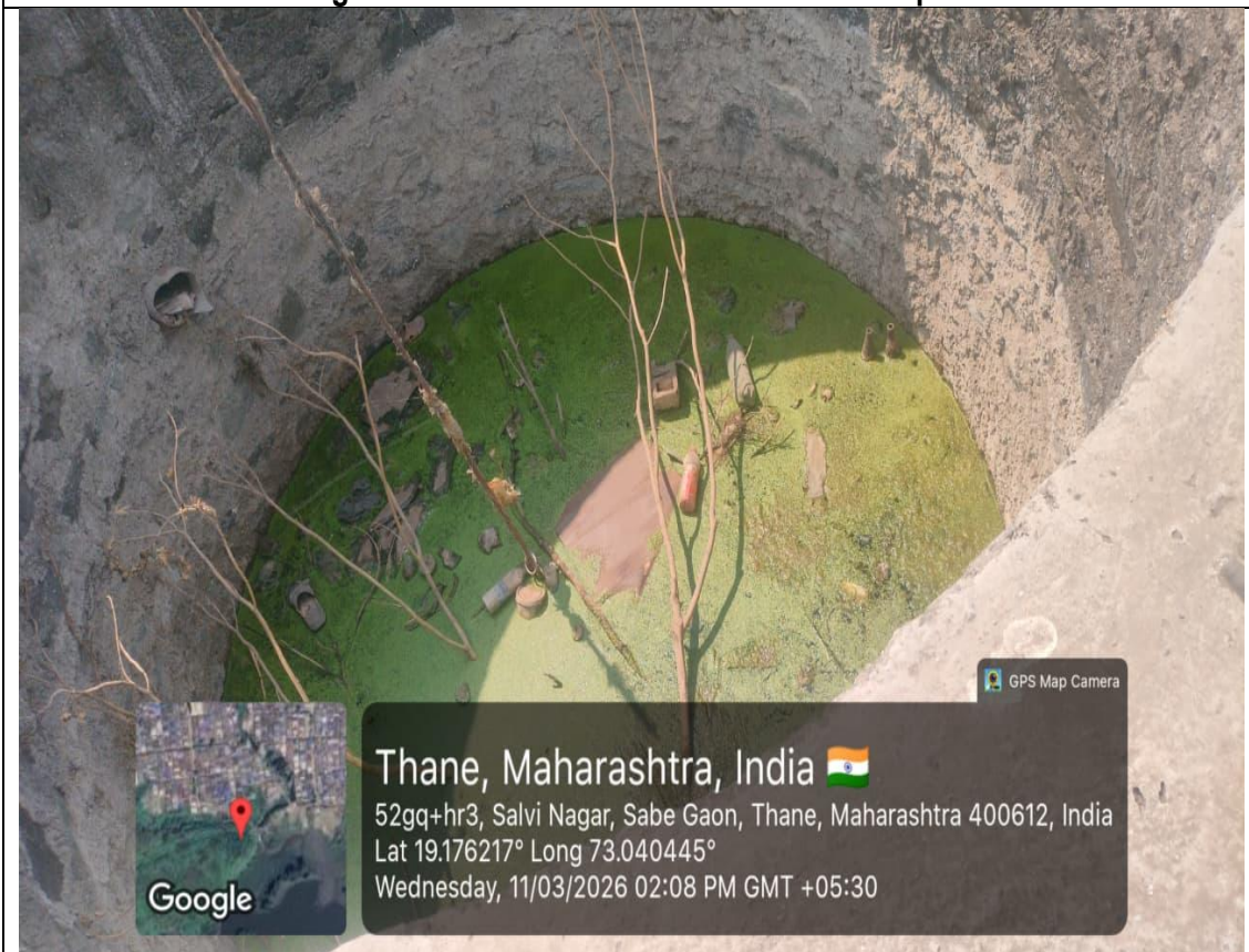
Image no 6: Wells for the collection of Leachate
